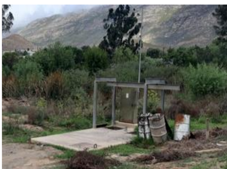
Pump station fencing: R136 000 Reservoir booster pumpstation: R380 00
